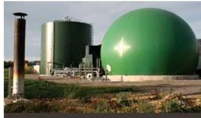
1480m 3 AD plant on a UK farm processing slurry, maize and glycerol.
